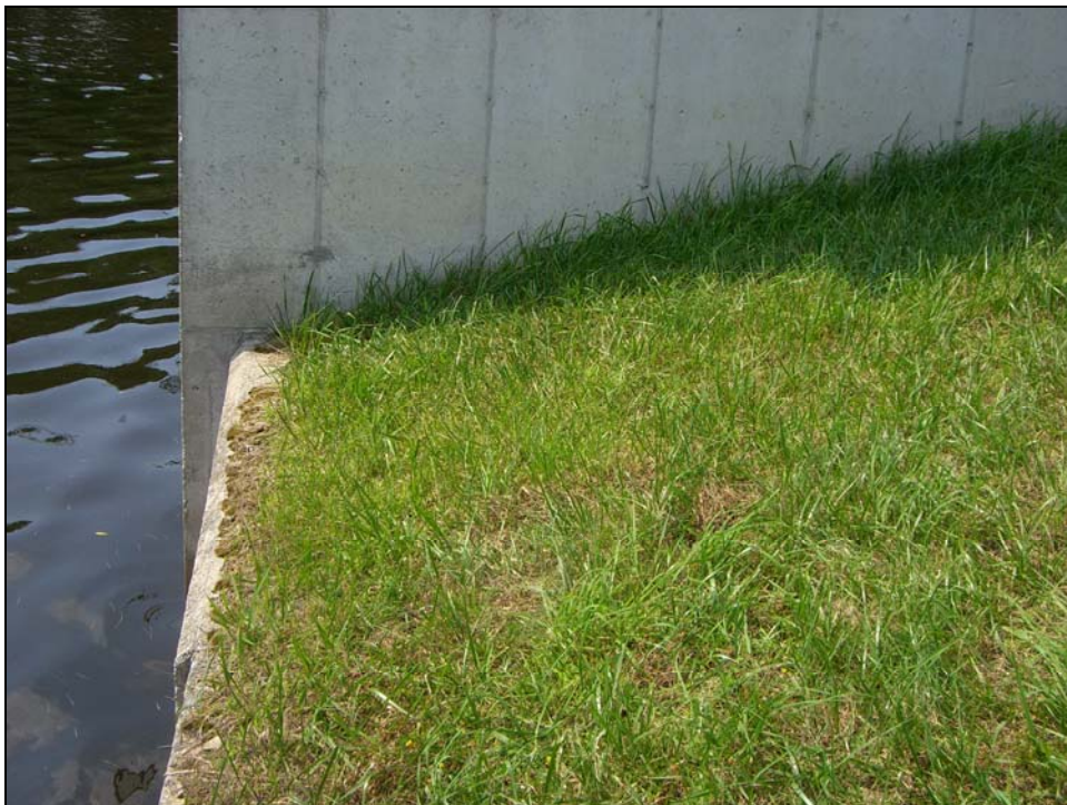
Photo 06 - The upstream wave wall and gatehouse foundation to the right of the primary spillway. Minor outward wave wall movement was observed in this area.
