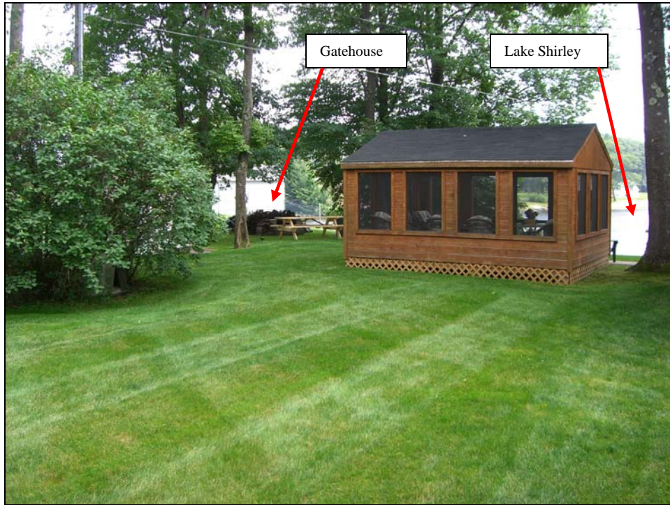
Photo 08 - The dam crest on the private property near the left abutment. Lake Shirley and the gatehouse are visible in the background. The crest is up to 120 ft. wide in this area.
