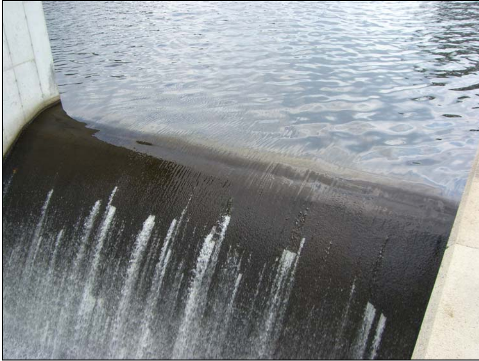
Photo 17 - A close-up of the ogee weir looking upstream. The minor flow interruptions observed on the weir are small spalled areas.
