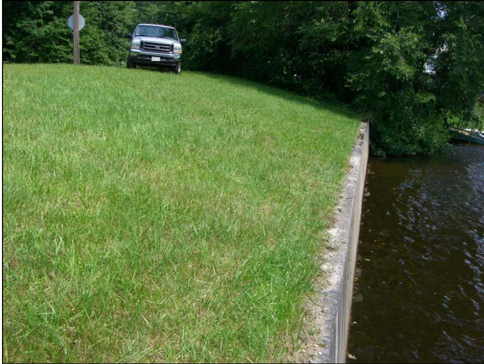
Photo 05 - The upstream slope to the right of the primary spillway. The trees and brush on the upstream slope are on private property. The grassed portion of the slope appears to be well maintained. The right abutment is beyond the truck and telephone pole in this image.
