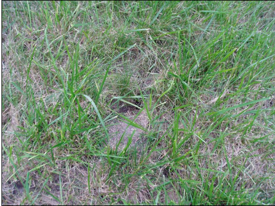
Photo 15 - A small animal burrow observed on the downstream slope to the right of the primary spillway.
