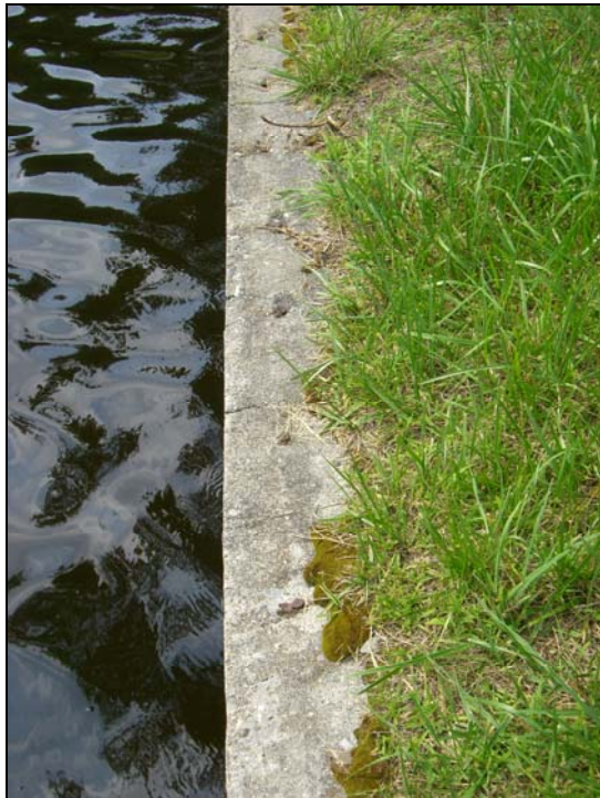
Photo 04 - The top of the wave wall to the left of the primary spillway looking to the left. The tops of cut off vertical steel bars are visible along the top of the wall.
