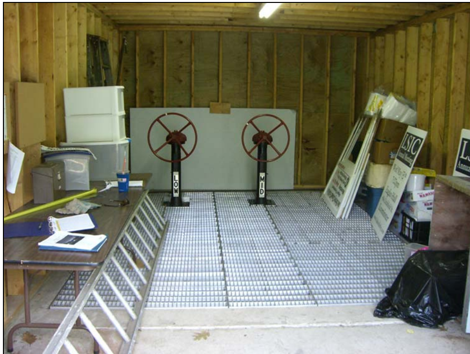
Photo 20 - The interior of the gatehouse structure with LLO and MLO hand wheel gate operators. The gatehouse and outlet works appear to be in satisfactory condition.
