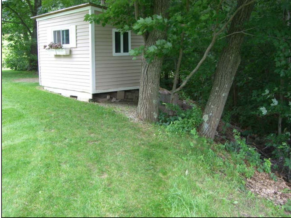
Photo 13 - The downstream slope looking towards the left abutment on private property. The slope near the left abutment is overgrown with trees and brush. However, the embankment crest is up to 120 ft. wide in this area.
