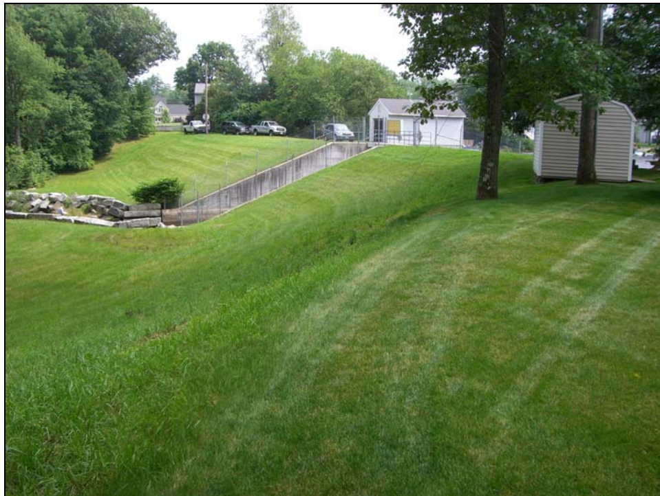
Photo 12 - The downstream slope looking towards the primary spillway from the private property near the left abutment. The grass is well maintained although some weeds were observed in this area.
