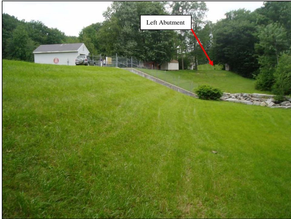
Photo 11 - The downstream slope looking towards the primary spillway from the right abutment area. The slope is surfaced with a well maintained grass cover. The left abutment is at the hill visible in the background of this photo.
