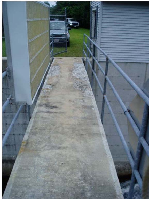
Photo 18 - The concrete catwalk looking towards the right side of the spillway. Spalling of the catwalk surface was observed.
