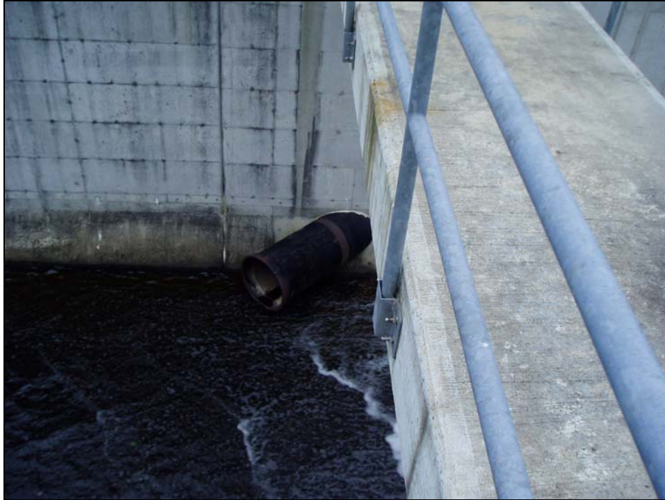
Photo 21 - The discharge pipe of the outlet works protruding from the right wall of the spillway discharge channel. No seepage or leakage was observed.
