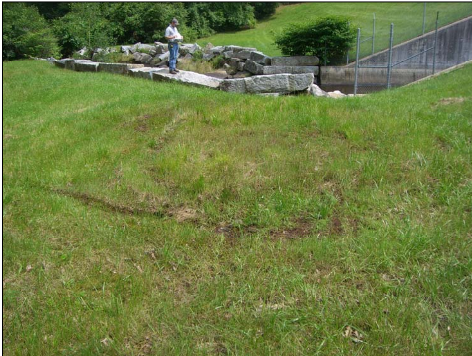
Photo 14 - A wet area was observed at the toe of the downstream slope to the left of the primary spillway. Standing water was observed but no active seepage was detected. There is a toe drain seepage collection system in this area. The drainage pipe of the system may be clogged resulting in this wet area.
