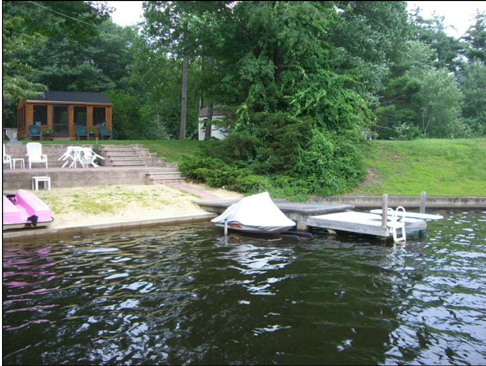
Photo 03 - The upstream slope and crest of the dam near the left abutment. This private home site may have been the site of a former mill. The site is essentially level with the embankment crest shown in Photo 02 and is between 40 ft. wide and up to approximately 120 ft. wide where the site contacts the left abutment.
