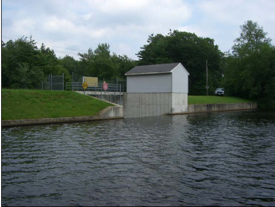
Photo 01 - The upstream slope/face of the dam. The primary spillway, gatehouse, concrete wave walls, and grassed earthen slope are visible in this image. The right abutment is beyond the truck and telephone pole in this image.
