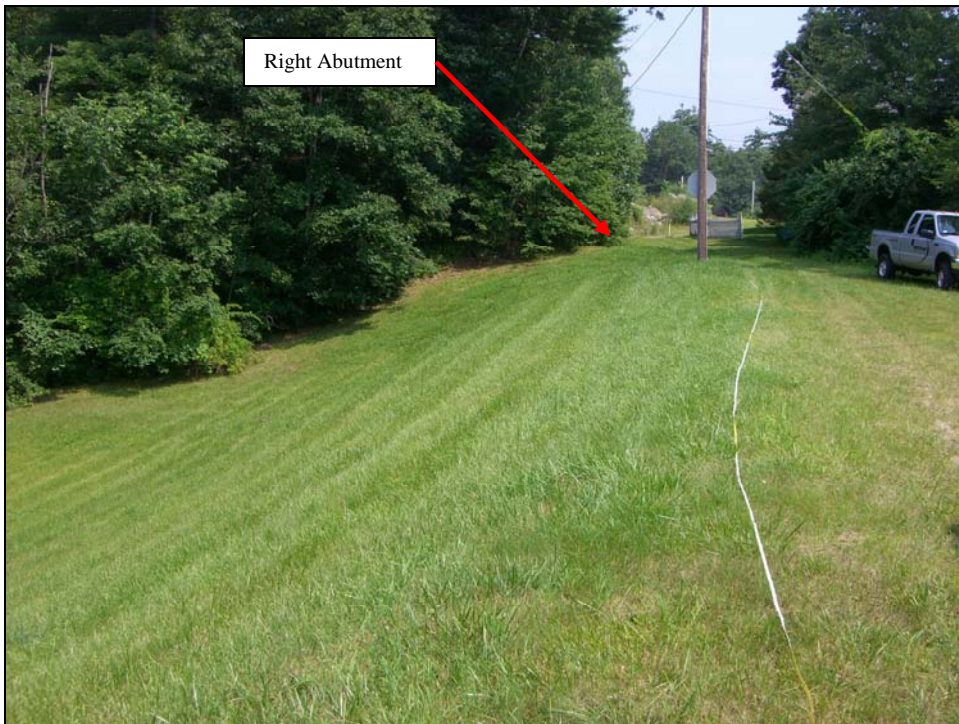
Photo 10 - The crest and downstream slope to the right of the primary spillway looking towards the right abutment. The crest and slope are surfaced with well maintained grass.
