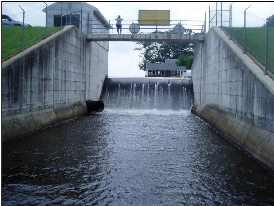
Photo 16 - The primary spillway looking upstream. The ogee weir, concrete catwalk, and discharge channel walls are visible. The minor flow interruptions observed on the weir are small spalled areas. The pipe protruding from the right channel wall (left side in this image) is the discharge pipe from the gatehouse outlet works.
