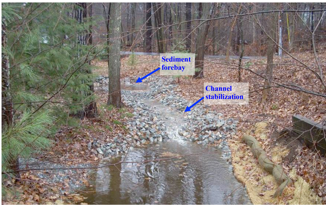
View upstream (towards Flat Hill Road) of newly constructed sediment forebay and stabilized channel section at 833 Flat Hill Road.
