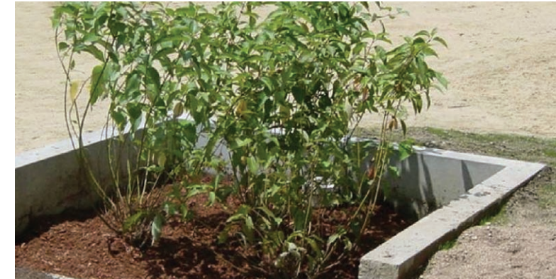
Filterra™ tree box filter installed to reduce pollutant loading to Long Lake (Littleton, MA).
