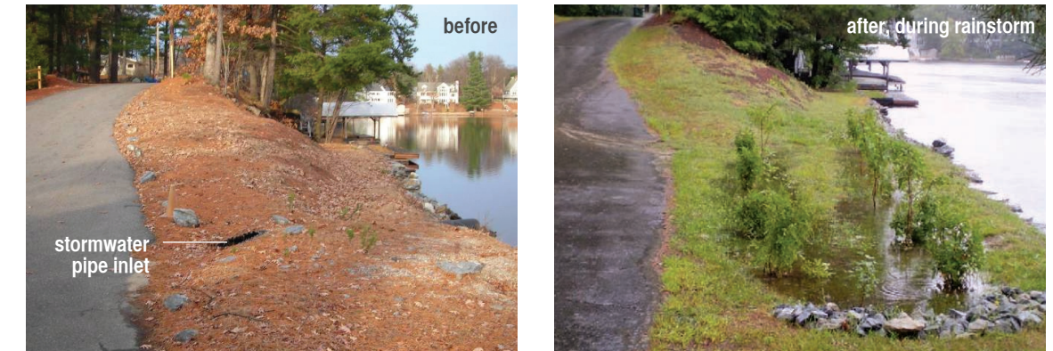
To eliminate a direct stormwater pipe discharge and reduce pollutant loading to Lake Shirley, a raingarden was installed to infiltrate and treat stormwater at the southern end of Sunset Lane.
